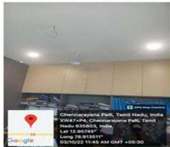
LED lights in the admin (office) room located in Admin block
