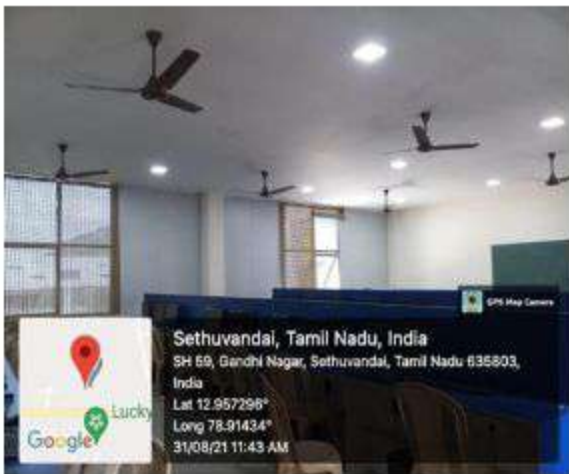
LED Lights in Computer Lab (Room No. 220)
