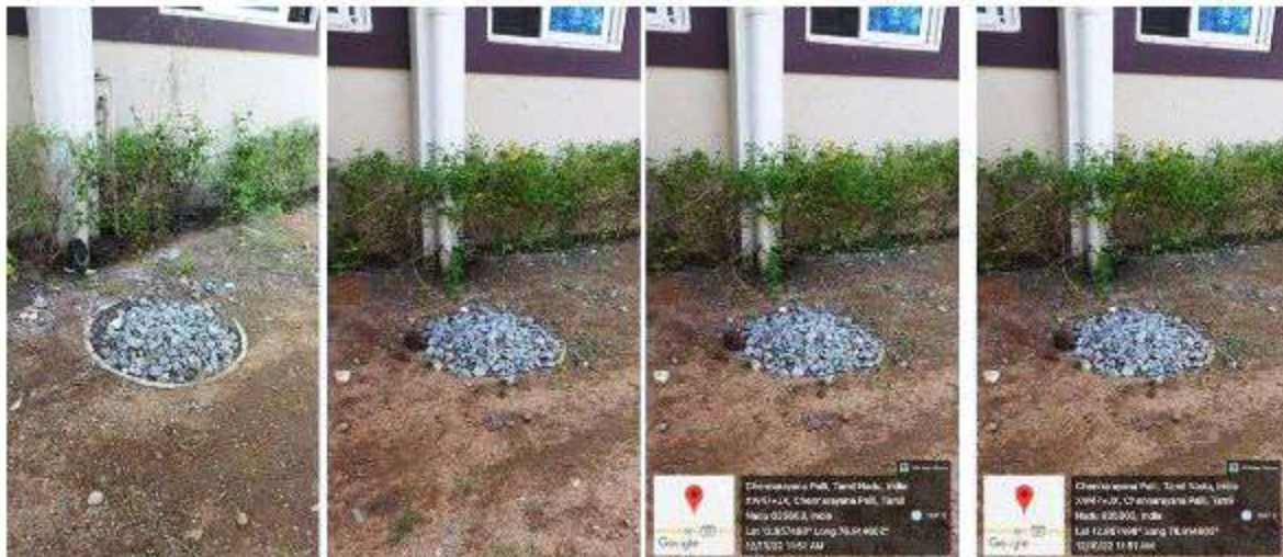
Water Conservation – Rain water harvesting
